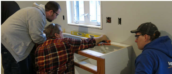
Saint Paul College cabinetry students installing new kitchen cabinets at 36th House
